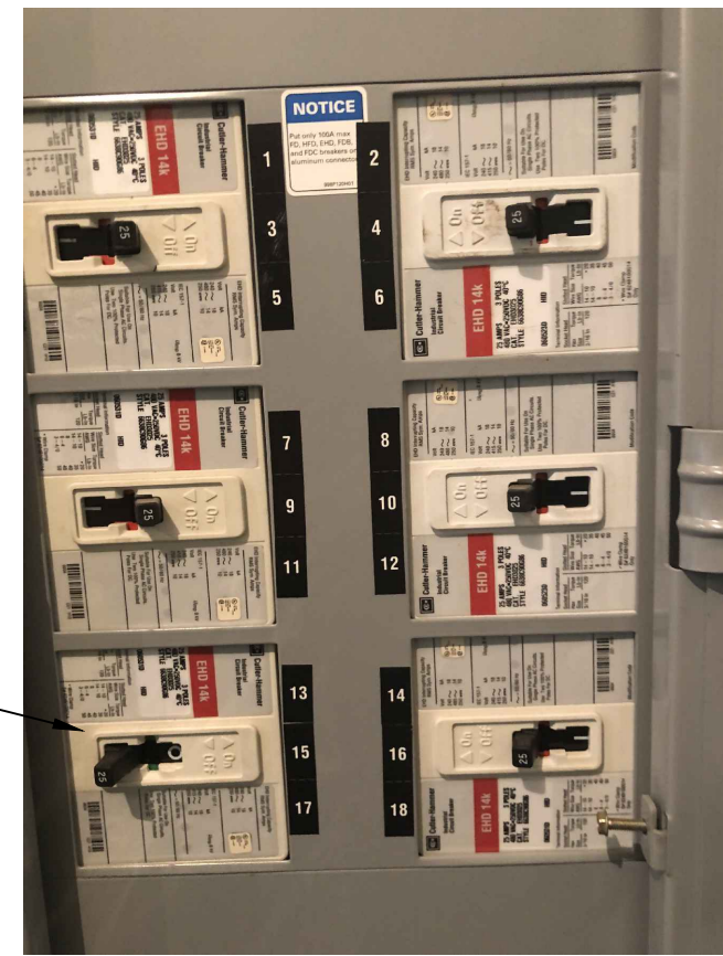
EXISTING POWER PANEL
