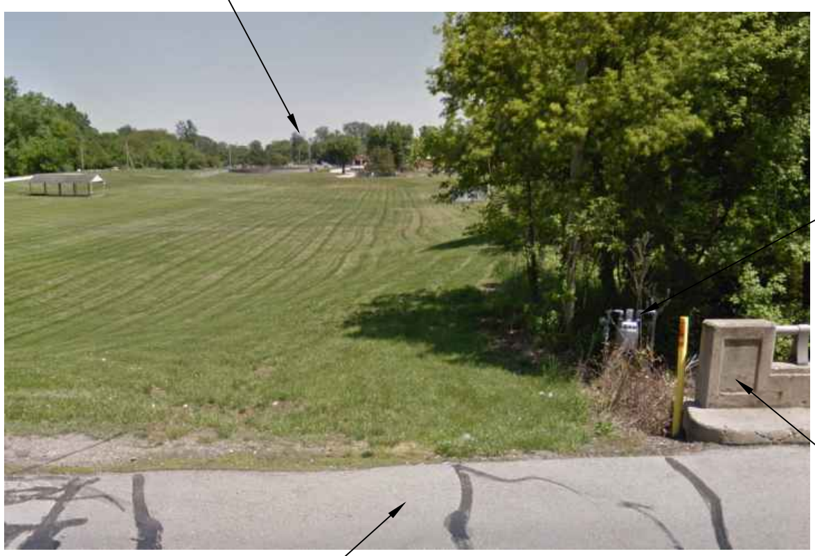
NATURAL GAS METER AND PRESSURE REGULATOR SET EAST SIDE OF BRIDGE GUARD RAIL OVER GREENVILLE CREEK
